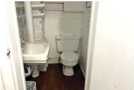
Restroom – not ADA compliant
