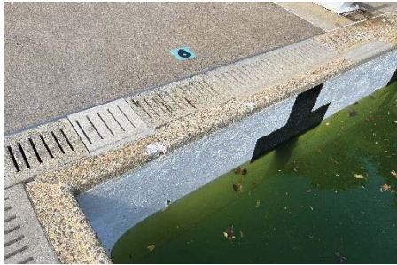
Broken, replaced, and worn coping
