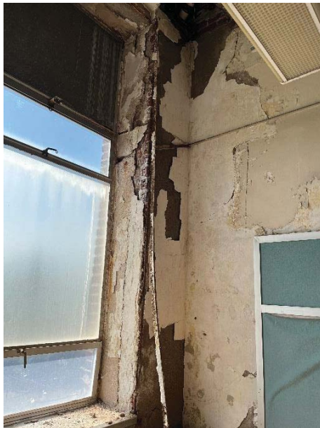
Original exterior masonry wall – view from inside showing destruction from water
