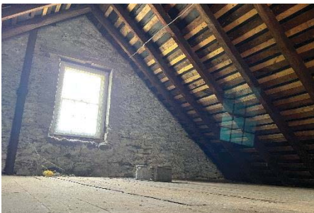
Uninsulated roof and walls
