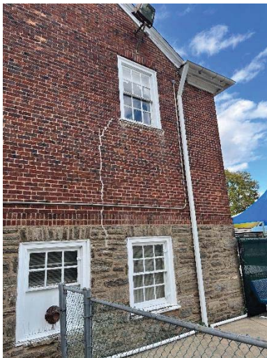
Structural cracks in masonry wall and single pane glass wood windows
