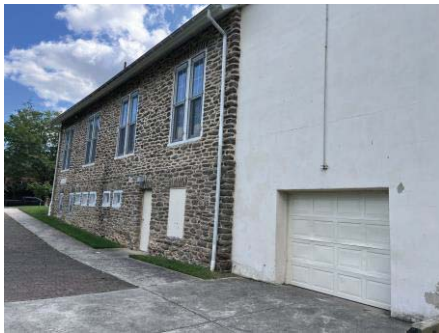
View of stone wall in need of cleaning and sealing, and condition of garage door
