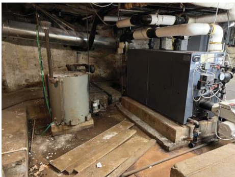
Mechanical systems in basement
