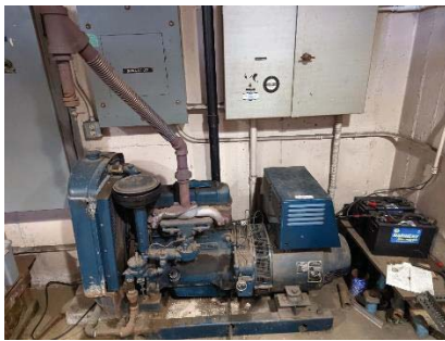
Kohler Emergency Generator
