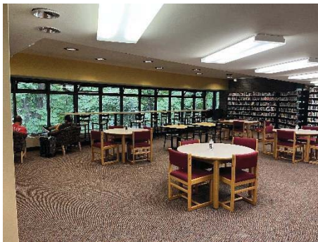
Photo showing condition of carpet
