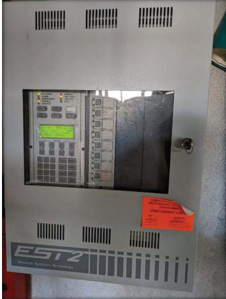
Edwards EST2 fire alarm control panel.
