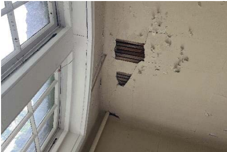
Plaster ceiling that has fallen leaving a hole In the ceiling – note peeling paint
