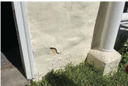
Delamination of paint from stucco
