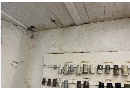
Wood ceilings in basement – shows evidence of water damage
