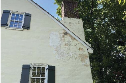
Issues at chimney
