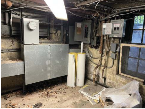
Electrical equipment amongst water piping
