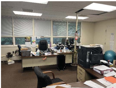
Ceiling tile with water stains
