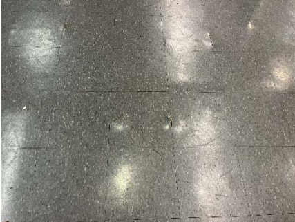
Condition of some VCT flooring
