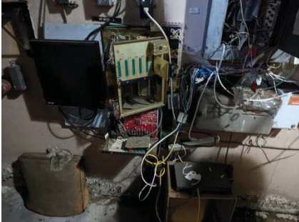
Telecomm Service Entrance
