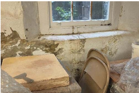
Water issues in basement
