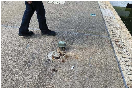
Electrical box sticking up is a trip hazard
