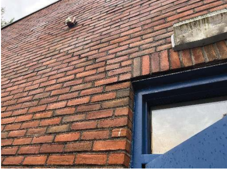
Crack in brick that extends from corner of door
