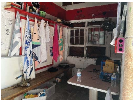
Open electrical box with exposed wires
