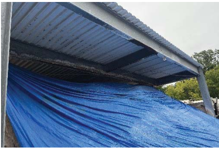
Rusted steel beams at salt shed
