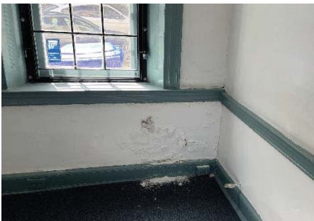
Water issues on interior and security gate on window
