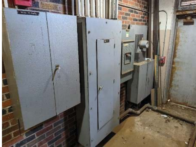
Main Distribution Panelboard
