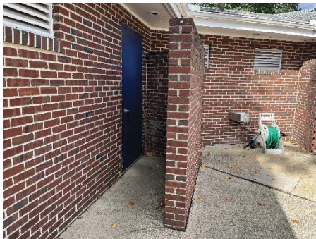
Entry into locker room does not meet code
