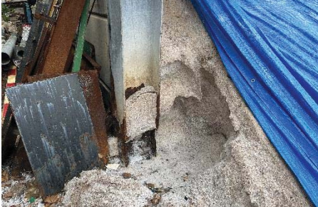
Rusted steel column at salt shed
