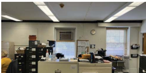
Example of exterior plaster walls in need of patching/refinishing
