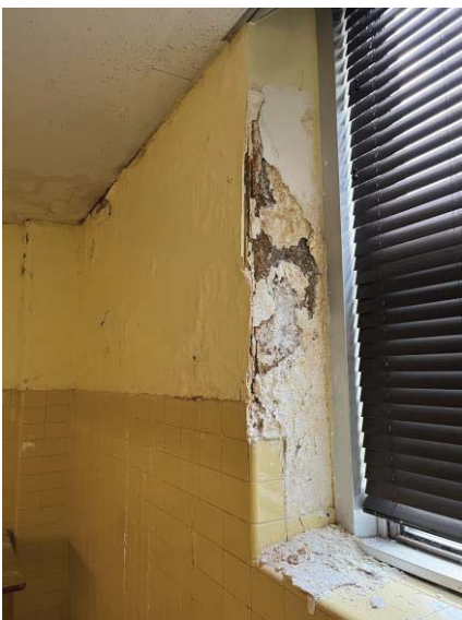
Example of water intrusion and the damage it is causing
