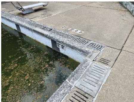
Same as above, and rusted diving board
