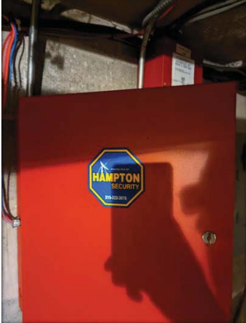
Fire alarm control panel
