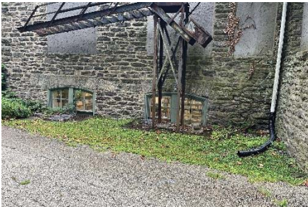
Rust egress stair from upper level
