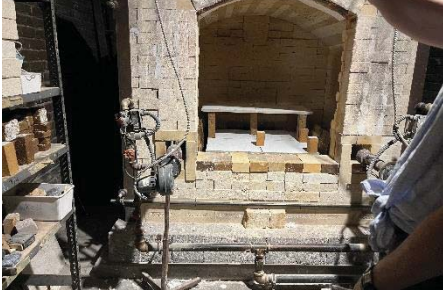
Open kiln in basement
