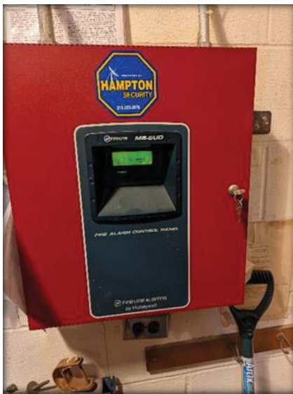
Firelite fire alarm control panel
