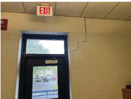
Crack in CMU block wall
