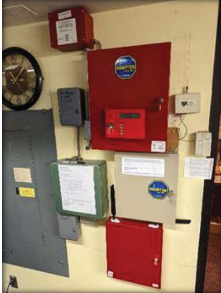
Fire/Security alarm control panel
