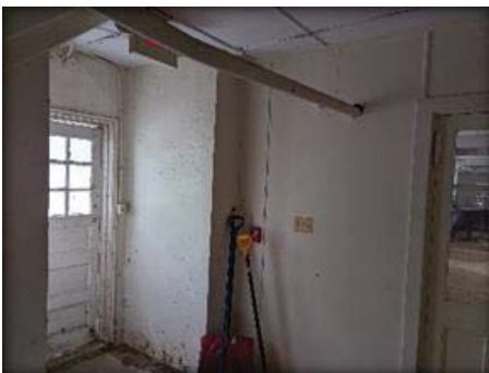
Exit sign in basement blocked by pipe
