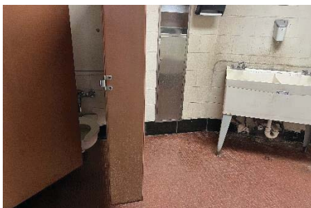
Restroom – not in compliance with ADA
