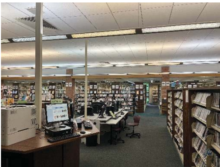
Discolored fluorescent lighting
