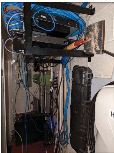
Enclosed data rack
