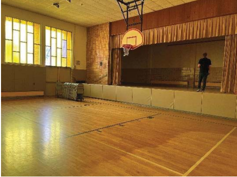
Code issues related to gym space include need to provide ADA access to the stage, replacement of all the single pane windows
