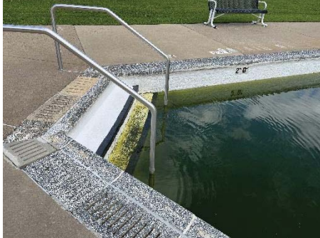
Example of pool coping, broken and with exposed aggregate
