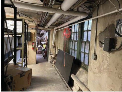
Various plumbing components in basement
