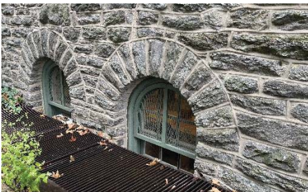
Crack in stone wall
