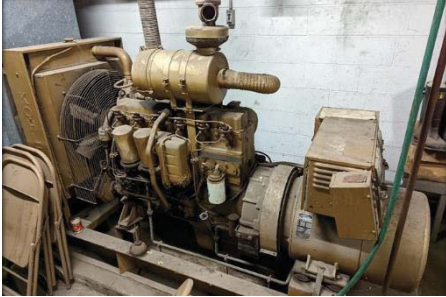
Kohler Emergency Generator
