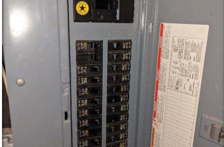
Main electrical panel board
