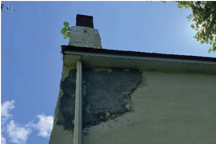
Issues at chimney
