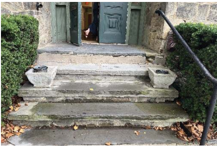
Masonry in need of repair
