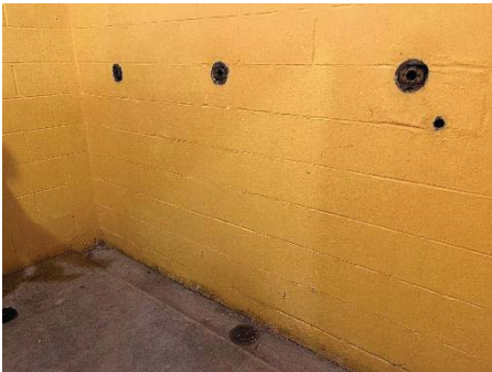
Showers with missing faucets and trench drains that are not permitted by code
