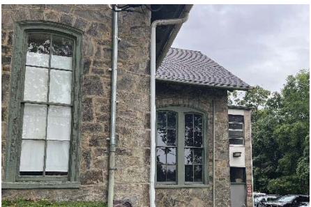
Window with peeling paint
