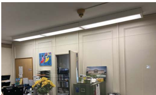
Example plaster ceiling with surface mounted light fixtures and wire molding
