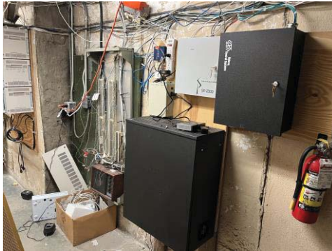
Phone and security panels
