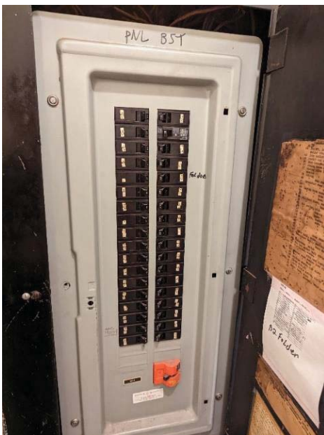
Existing Panelboard in basement with cloth insulated conductors
