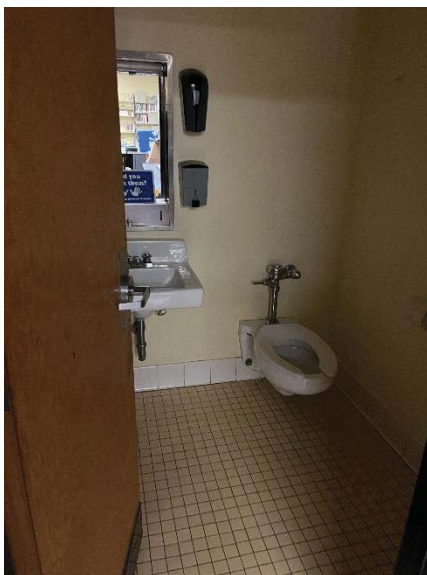
Photo of non-compliant restroom
