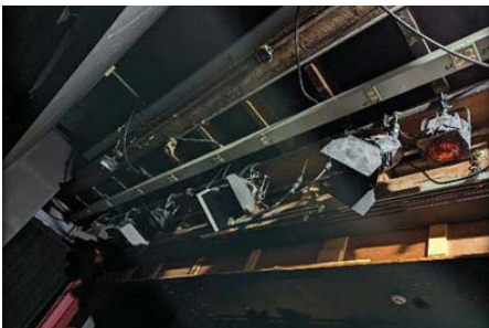
Existing theater lighting
